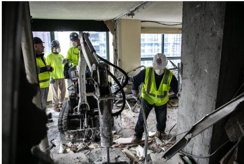
Construction workers demolishing the upper floors of the DoubleTree Suites at 1568 Broadway, which closed in February. Jeenah Moon for The New York Times
