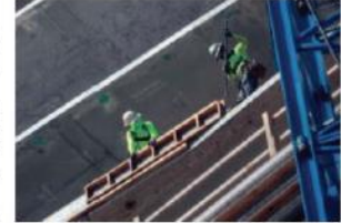
Workers remove concrete molds as work continues on One West Palm, billionaire real estate developer Jeff Greene's twin-tower complex in downtown West Palm Beach on Nov. 22. LANNIS WATERS/PALM BEACH POST
