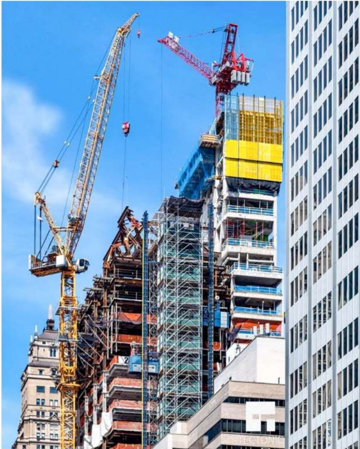
Closeup of the transition into the third section at 425 Park Avenue, by Tectonic
